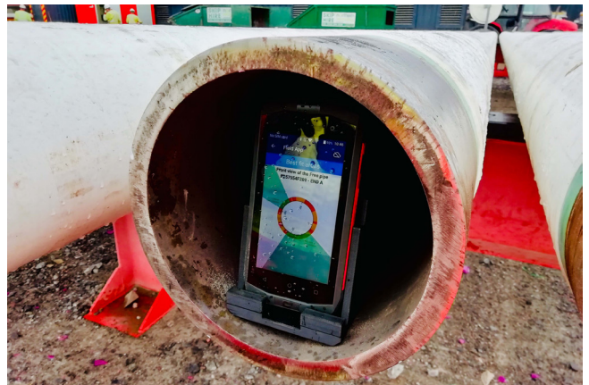
Figure 7. If pipe rotation is to be considered, the application will display the compatibility area along the circumference.
