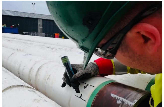
Figure 6. Based on the Best-Fit-Finder recommendations, welders mark accordingly the compatibility areas on the pipe OD.
