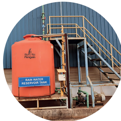
⬆ Rainwater recovery tank, Indonesia
